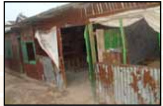
This classroom at Congo Town needs to be built from concrete.
